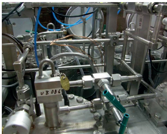
FIG. 10.14. A glimpse into a glovebox. The primary system consists of all-metal systems. Exceptions should be made only if it is absolutely necessary!
